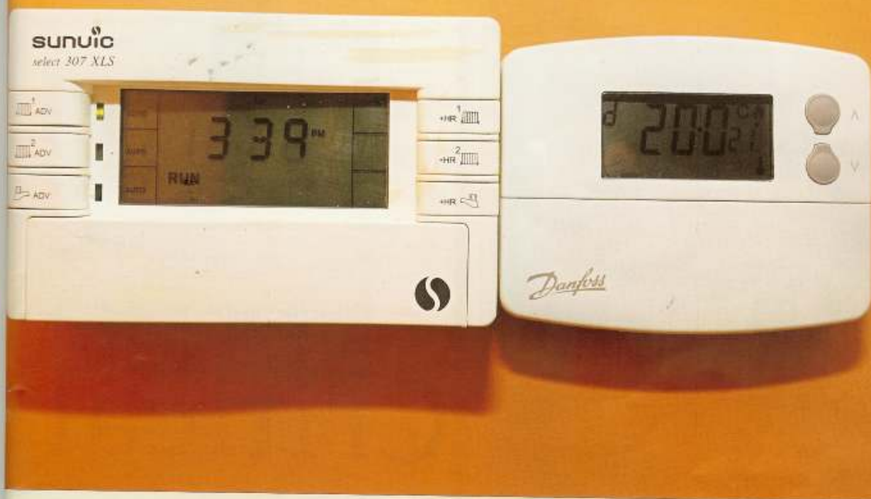
Also included in Kenny's upgrade was a Grant Vortex oil combi boiler (below) and heating controls to ensure that the house is heated efficiently (above)
